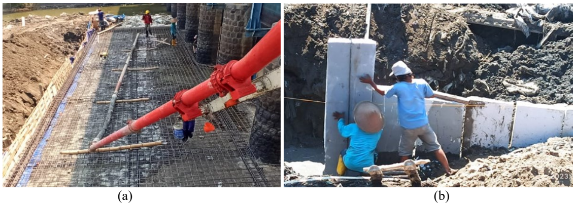
Figure 11. (a) construction of upstream floor strengthening and (b) installation of barrier wall
