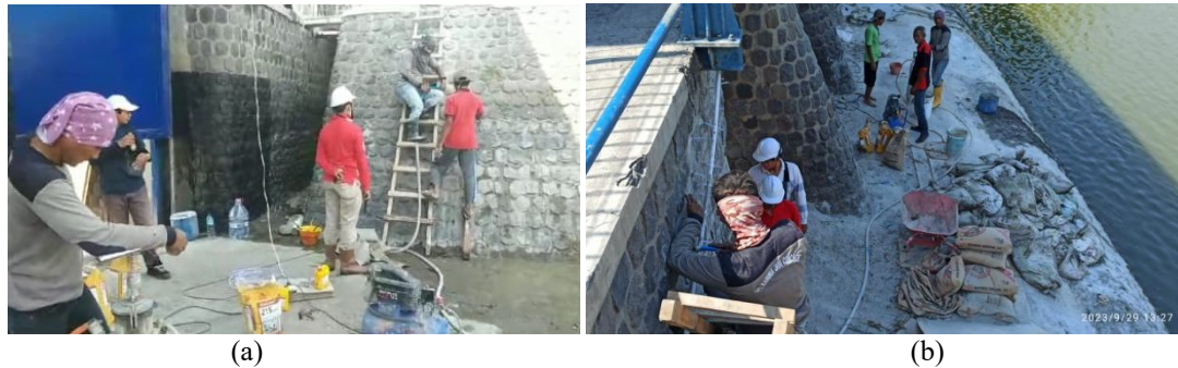
Figure 13. (a) grouting process of the stone masonry wall and (b) grouting process of the floor
